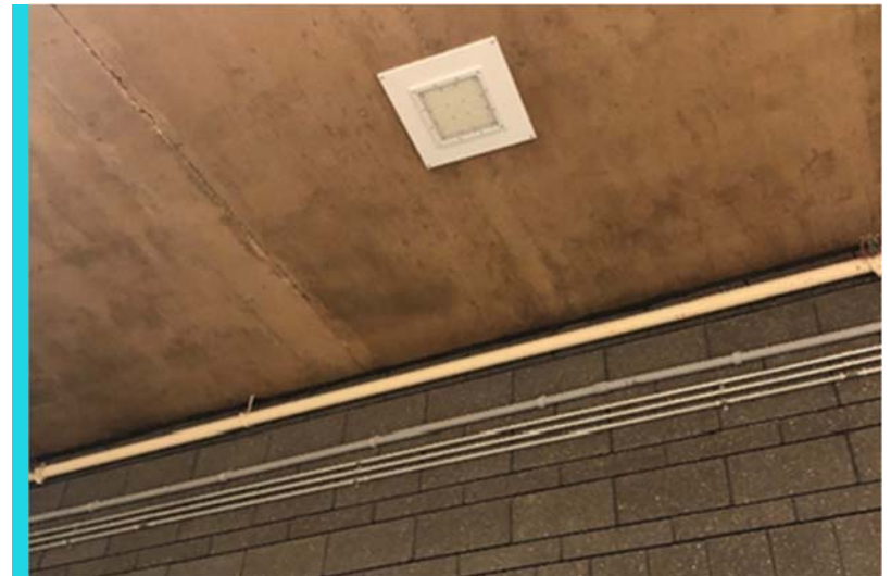
Fig. 55 - Damaged Soffit Source: Dialog
