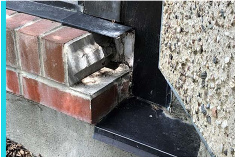
Fig. 37 - Exterior Brick Damage at Windowsill Source: Dialog
