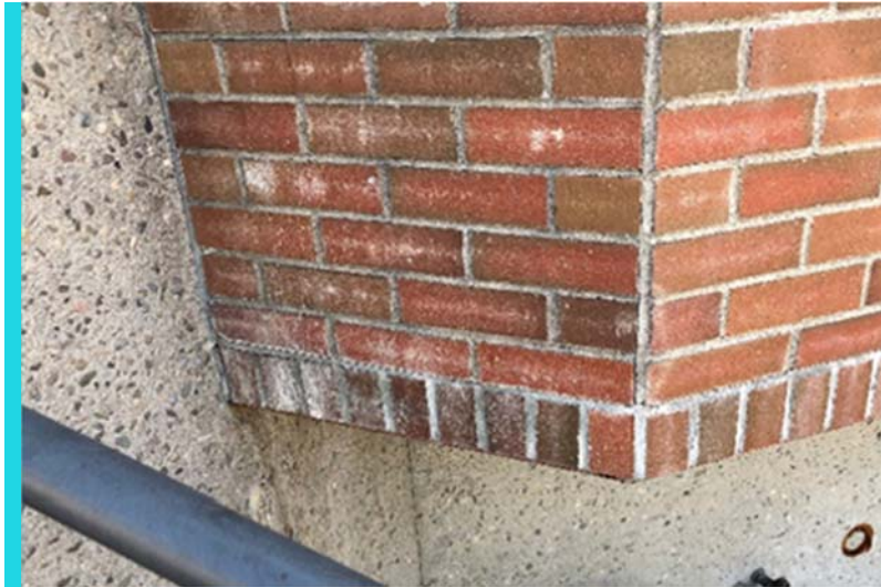
Fig. 41 - Exterior Brick Damage and Efflorescence Source: Dialog
