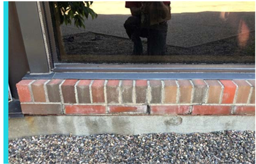
Fig. 35 - Exterior Brick Damage at Windowsill Source: Dialog
