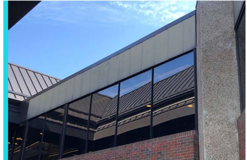
Fig. 43 - Damage at Exterior Wall and Fascia Source: Dialog
