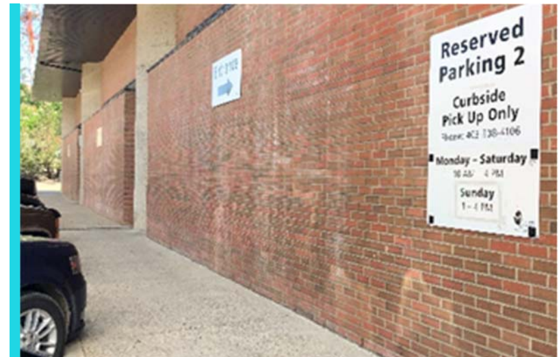
Fig. 36 - Exterior Brick Efflorescence Source: Dialog
