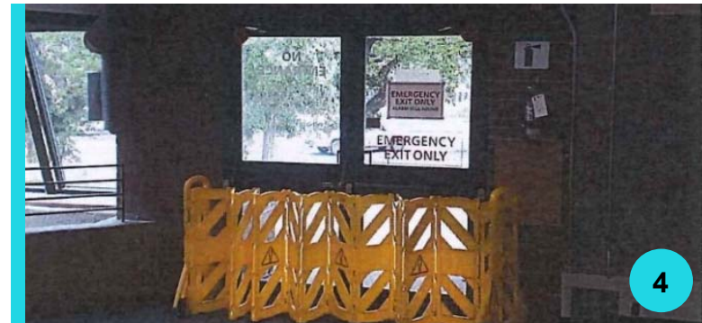
Fig. 96 - Blocked Entrance to North Wing from Stafford Drive South – Upper Level Source: RPG
