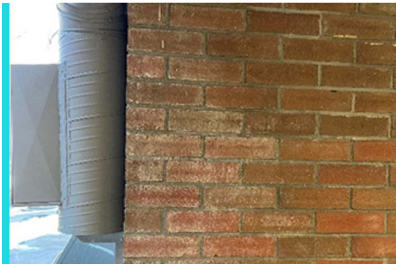
Fig. 42 - Exterior Brick Damage Source: Dialog
