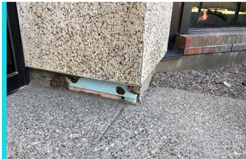
Fig. 34 - Exterior Cladding Damage at Wall Base Source: Dialog
