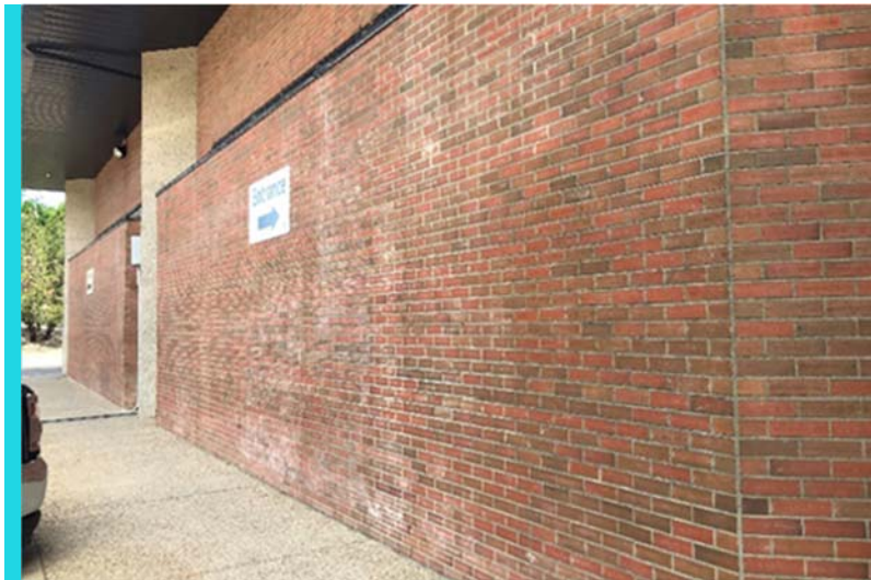
Fig. 38 - Exterior Brick Efflorescence Source: Dialog
