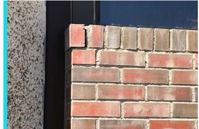
Fig. 39 - Exterior Brick Damage at Windowsill Source: Dialog
